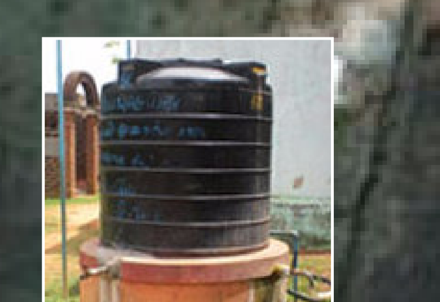
Tank and Pump
