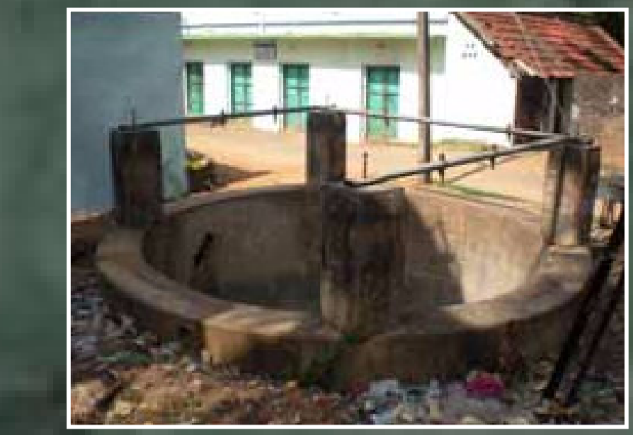
Well (not in use)
